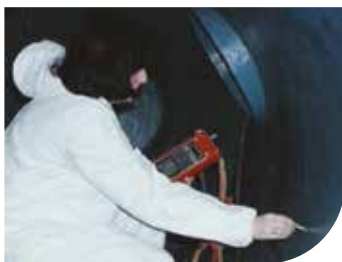
Chem-glass™ RA 200 Chemical Process Tank
