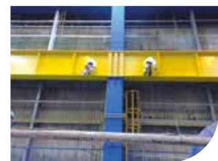
Easi-gloss™ RX 500GS Turbine Hall Structure
