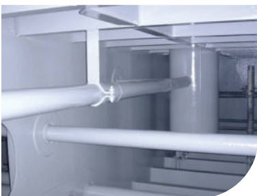
Diesel Fuel Tank
