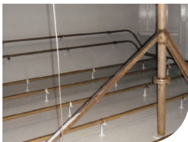
Crude Oil Tank
